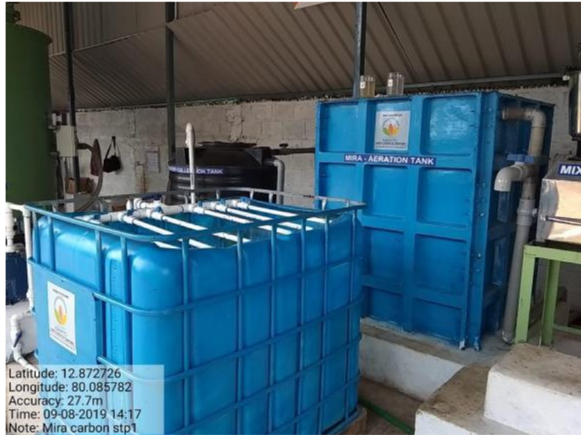
Mira carbon sewage treatment plant & Vermi flitration treatment unit
