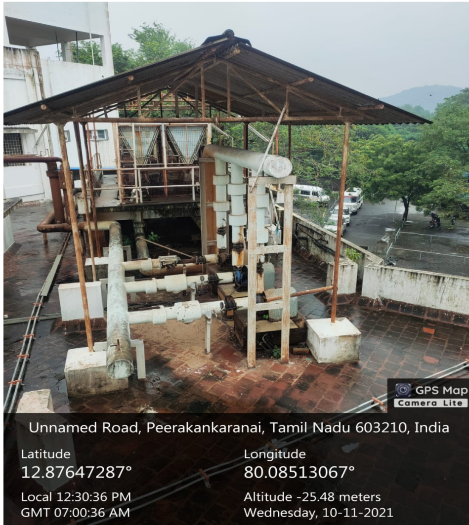
AIR-COOLED CHILLER PLANT
