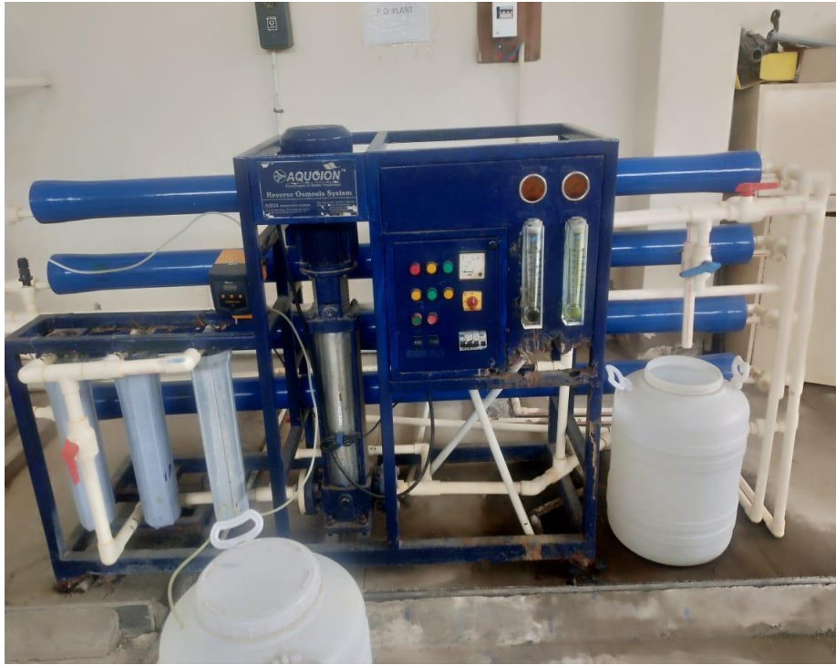
KBA MEN'S HOSTEL RO PLANT
