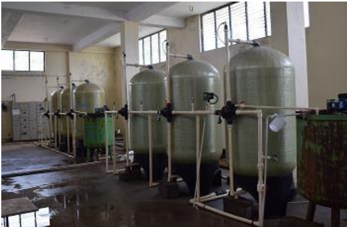
WATER TREATMENT PLANT
