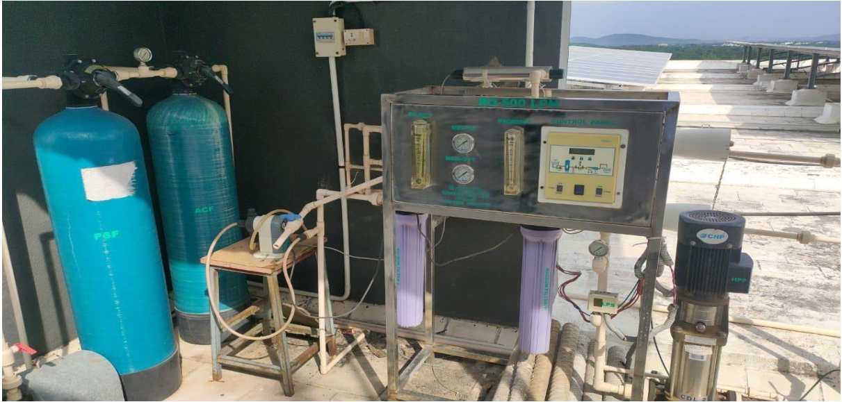
AERONAUTICAL BLOCK RO PLANT
