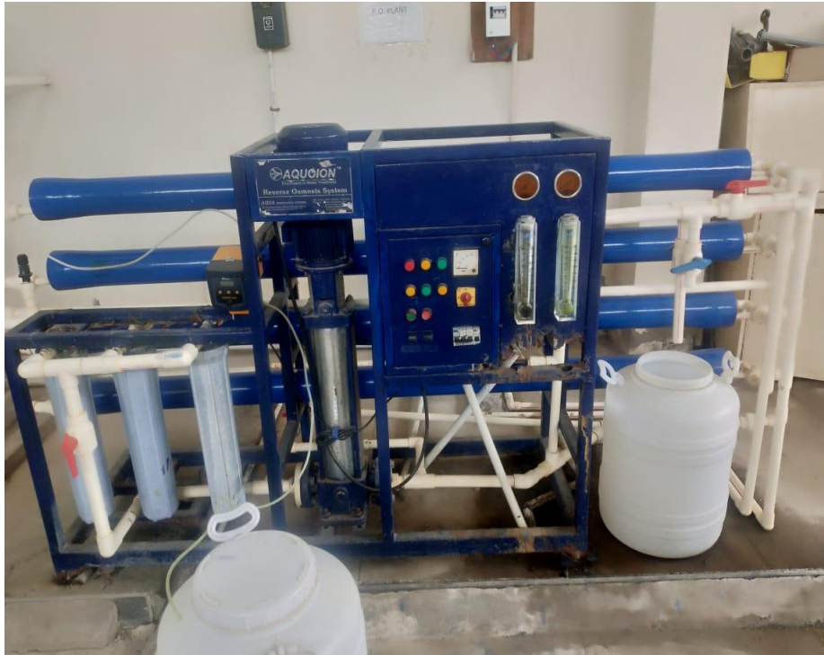
KBA MEN'S HOSTEL RO PLANT
