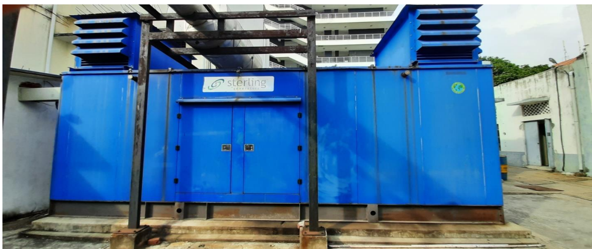
OUTDOOR DIESEL POWERED GENERATOR OF 750 KVA
