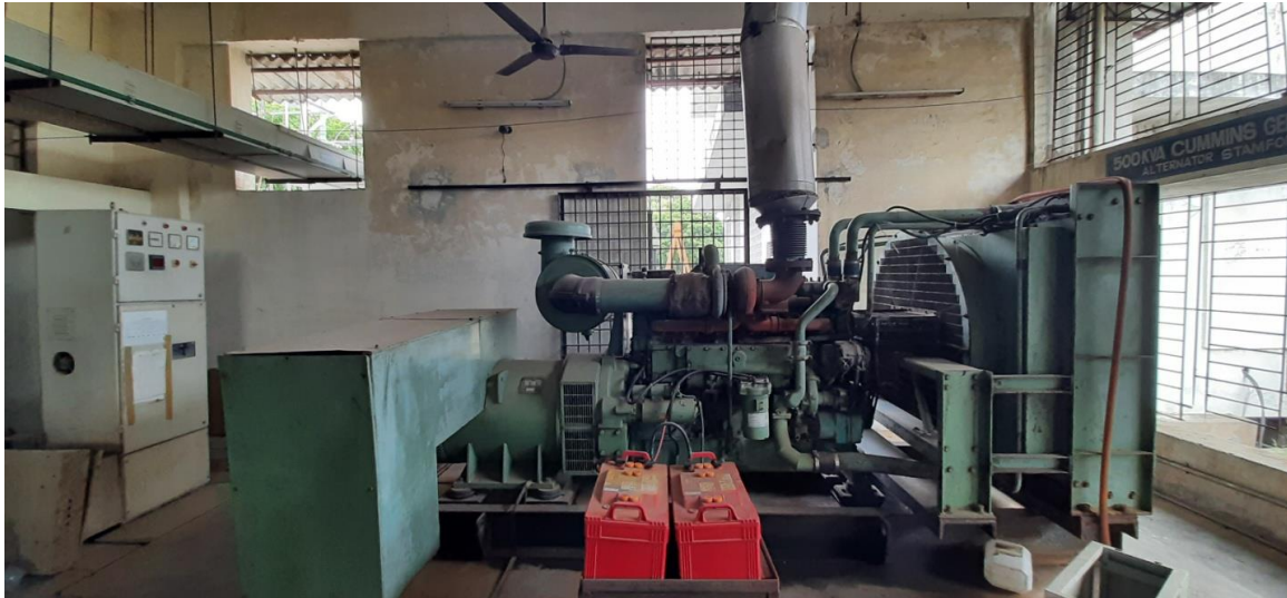
INDOOR DIESEL POWERED GENERATORS OF 500 KVA
