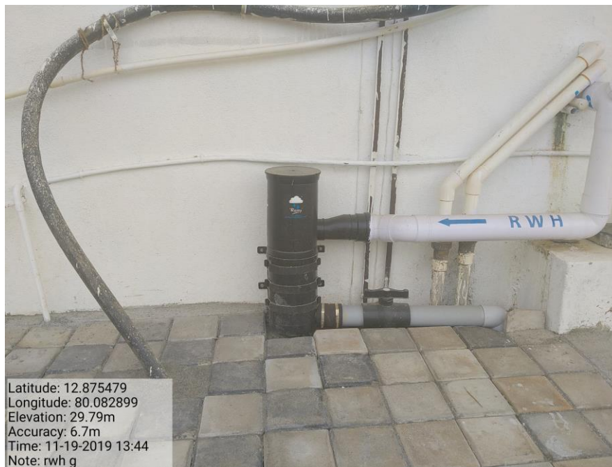
FILTER UNIT IN RAINWATER HARVESTING SYSTEM (ARCHITECTURAL BLOCK)
