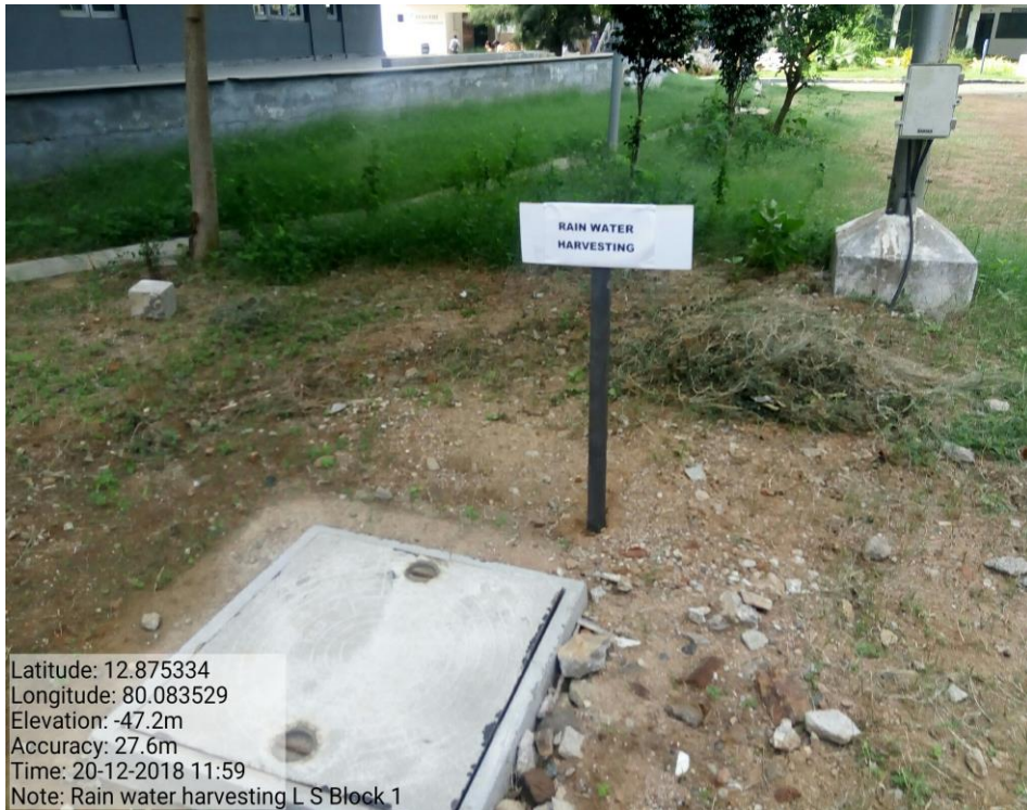
RAINWATER HARVESTING PIT AT LIFE SCIENCE BLOCK
