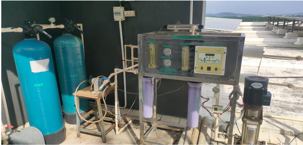
AERONAUTICAL BLOCK RO PLANT
