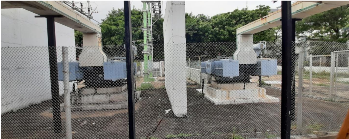
11 KV HT POWER SUPPLY / 8 00 KVA TRANSFORMERS
