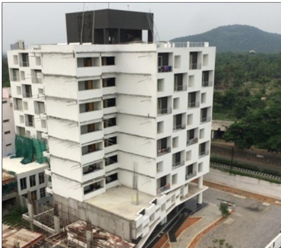
New Ladies Hostel Building (2015) Built up Area: 80000 sft. (G+7) Project Cost: Rs. 16.5 Crores
